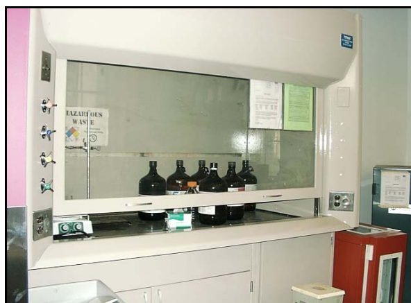
Typical Exhaust Hood
